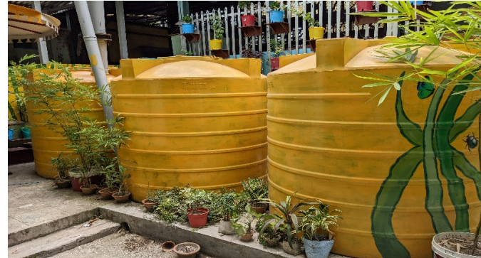
Rain Water Harvesting at Liluah Division
