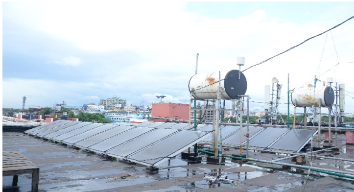
Solar Water Heater at Howrah Station /ER
