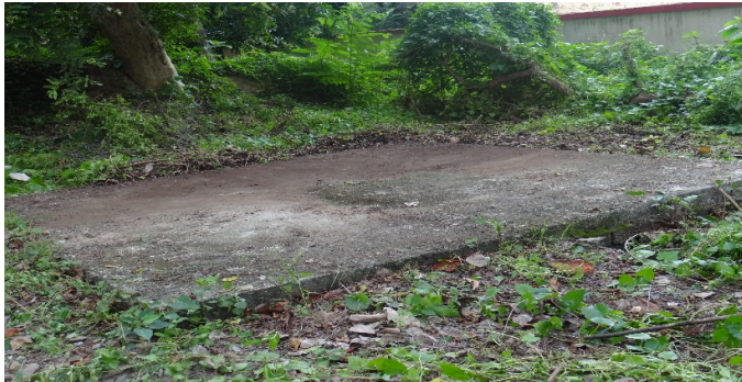
Rain Water Harvesting at Malda Division
