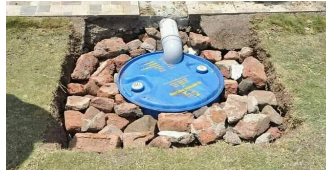
Rain Water Harvesting at Sealdah Division
