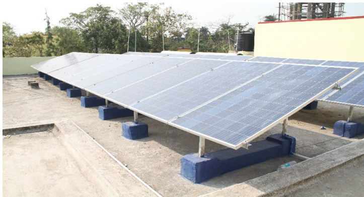
Solar Water Heater at Sealdah Station /ER
