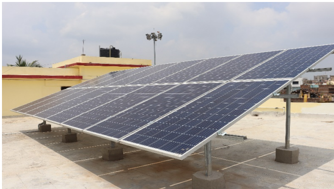
Roof top solar plant Bhagalpur Station/MLDT/ER
