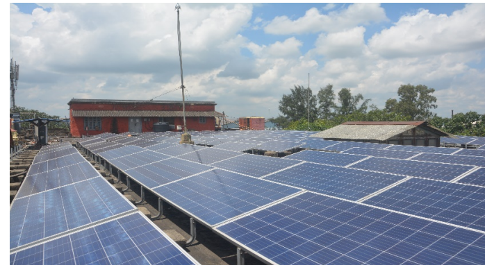
Roof top solar power plant Liluah Workshop/ER
