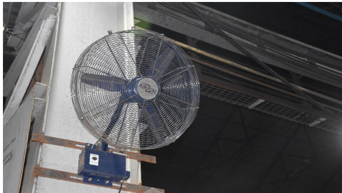
BLDC fans fitted in JMPW
