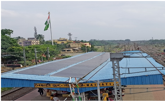
Roof top solar power plant Naihati Station/SDAH/ER
