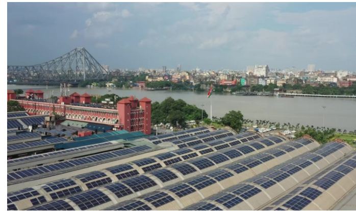
Roof top solar power plant Howrah Station/HWH/ER
