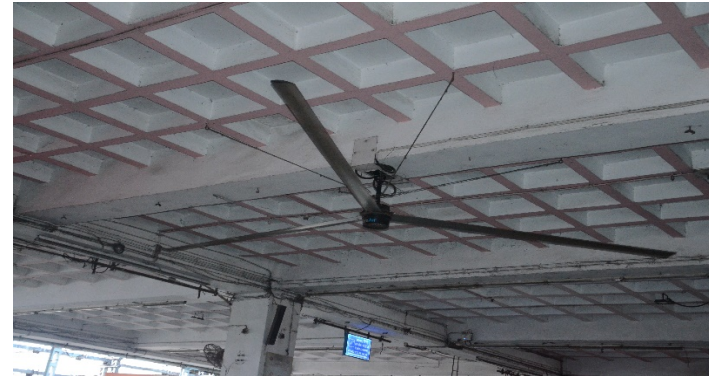
HVLS fans at Howrah division
