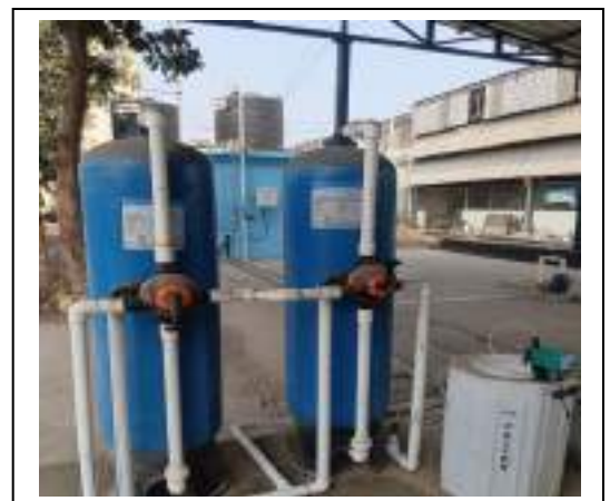
Filtration System with pressure sand &
