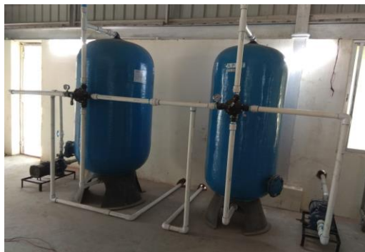
Water softener Plant
