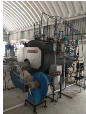
Industrial Big Boiler
