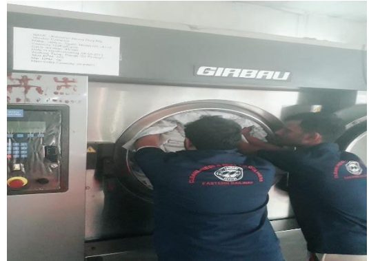
Loading of linen in washer cum extractor
