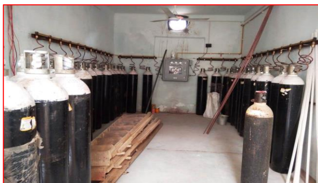
Manifold with Automated Panel and D Type Jumbo Oxygen Cylinders
