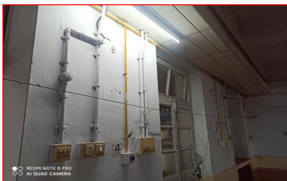
Oxygen Supply through Central Pipeline in Wards for Treatment of COVID - 19
