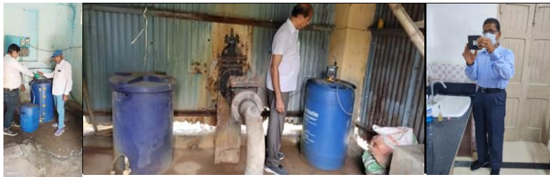
Chlorination Checking at Chlorination point BWN and BMG, Residual Chlorine Checking at RPH
