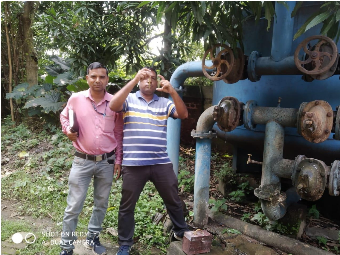
Residual Chlorine water testing at Filter House, Sitarampur
