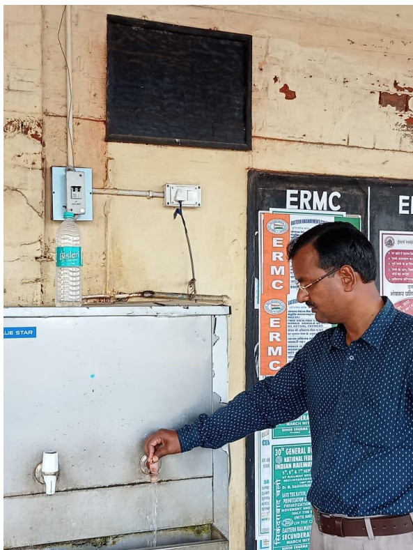
Drinking water cooler working, Panagarh Station
