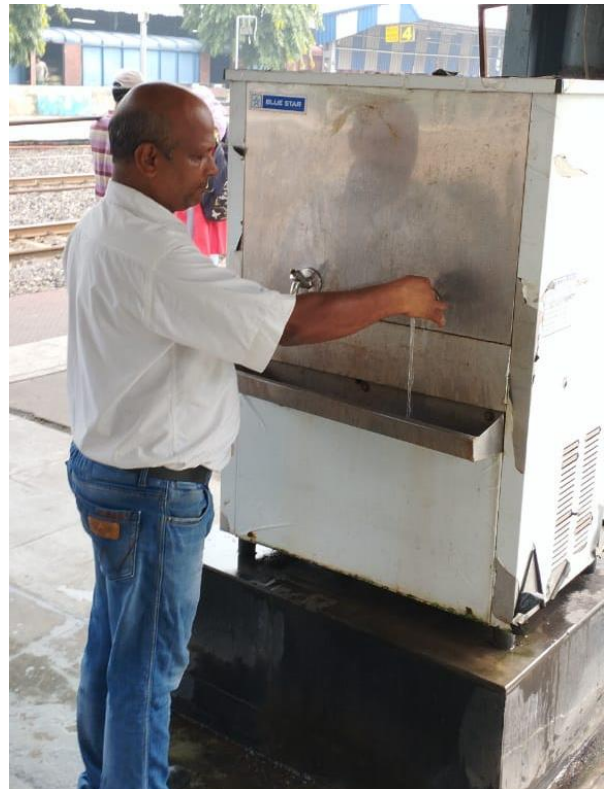
Drinking water cooler working, Durgapur Station
