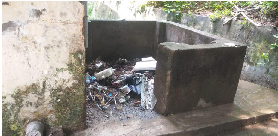
Garbage disposal at Divl. Rly Hospital, Asansol
