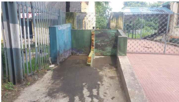
Garbage disposal at. Rly Hospital, Andal
