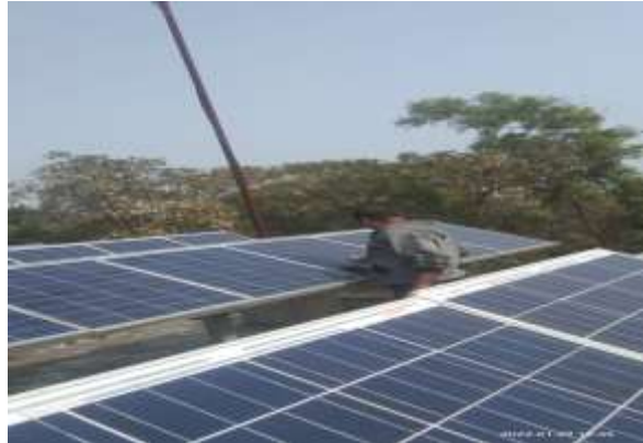
Solar Plant Gangatikuri
