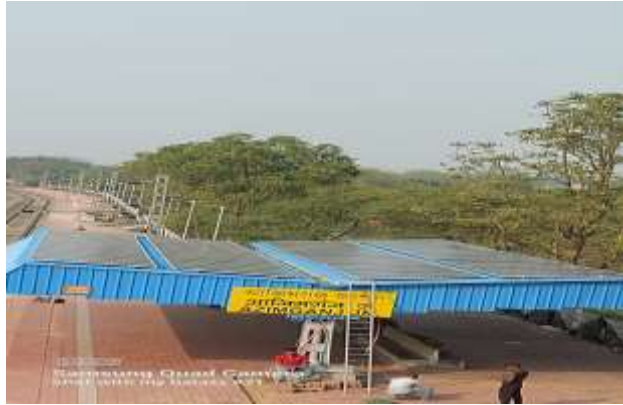
Solar Plant at Azimganj
