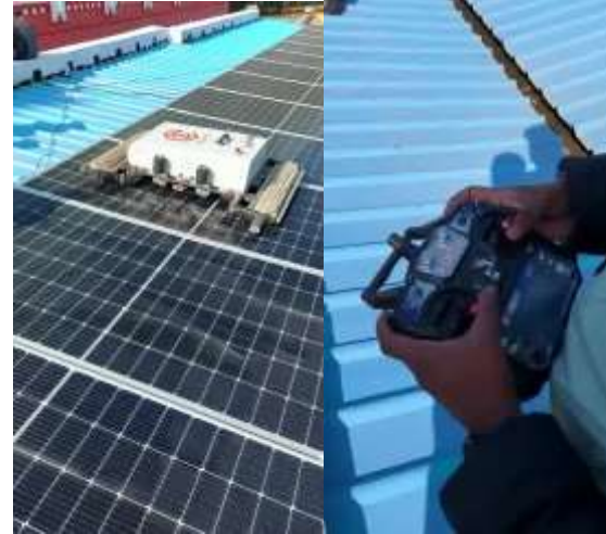
Robotic cleaning at Azimganj Solar Plant
