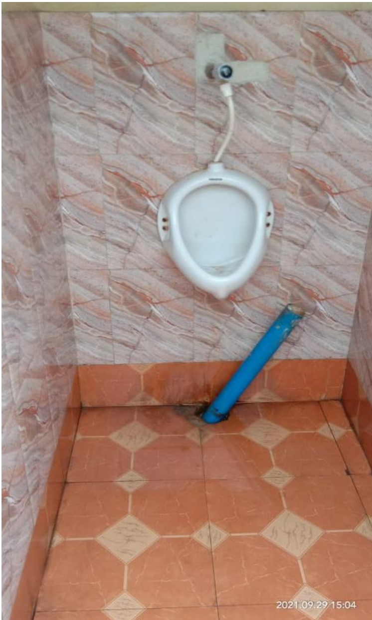
Before Repairing Urinal Pipe at Panagarh Station
