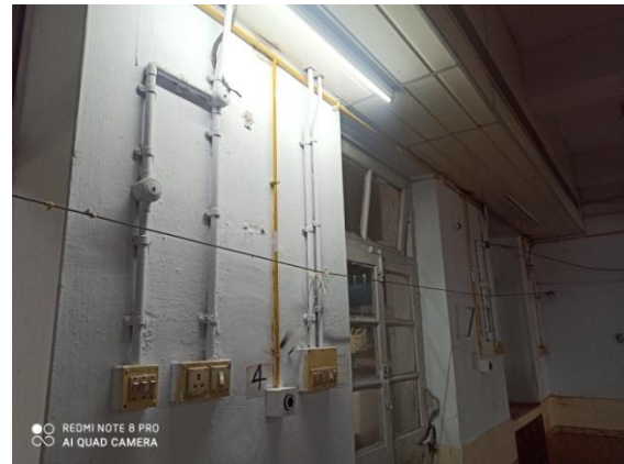
Ward with Central Gas Pipeline
