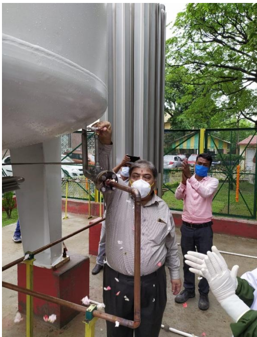
Commissioning of LMO Storage System by PCMD/ER on 16.04.2021
