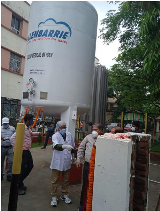
LMO Storage System
