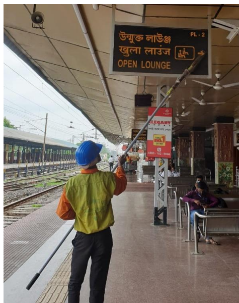
Before cleaning ceiling of open lounge area of Asansol Station on 25.09.2020
