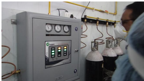
Manifold for Central Gas pipeline
