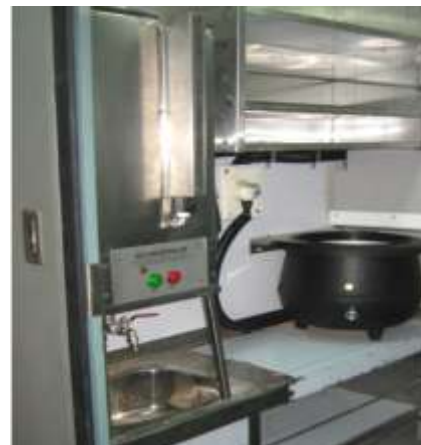
Vertical Water Boiler in Existing Design Coaches
