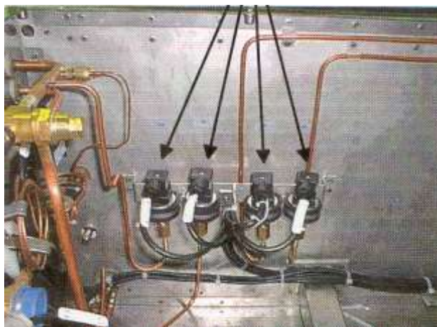
Figure 6.14 Pressure Transducers in RMPU
