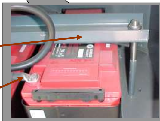
Battery Module Details
