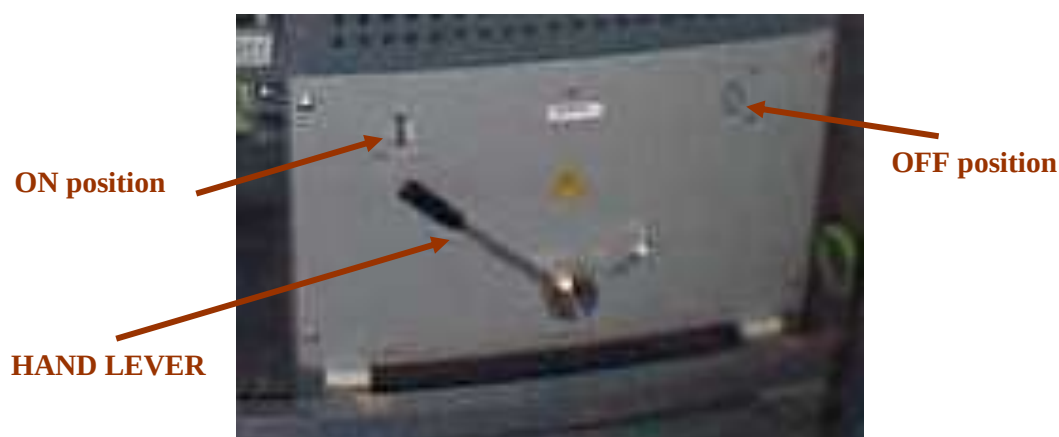
Figure 6.8 Disconnecting and Earthing Device
