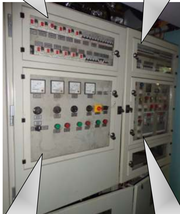
Switch board control panel
