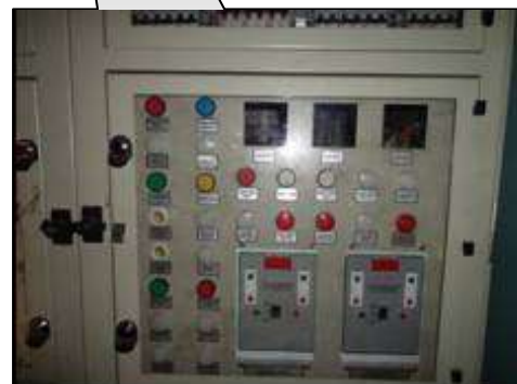
Control unit for water pump
