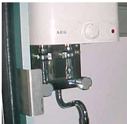
Figure 7.8 Water Boiler in Original design Coaches
