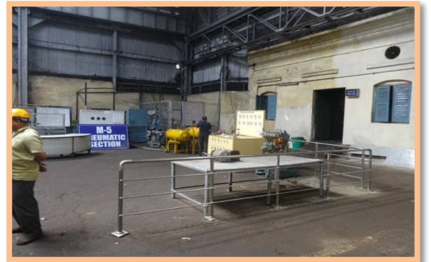
M-5 section after fitment of solar pipe lighting. Illumination=320 Lux.
