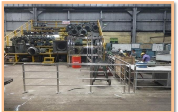
Auxiliary park after fitment of solar pipe lighting. Illumination=320 Lux.
