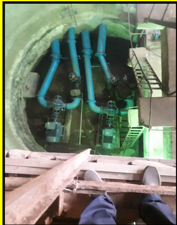
New Energy Efficient Pump
