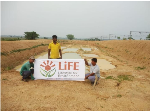
Artificial pond at Dubrajpur for Rain water harvesting
