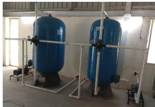
Water softener Plant
