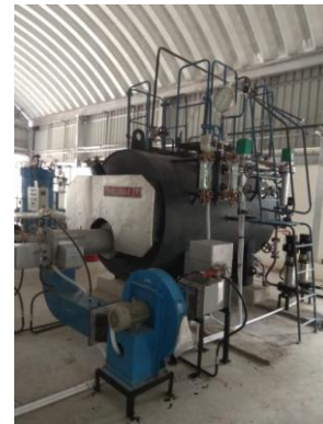
Industrial Big Boiler
