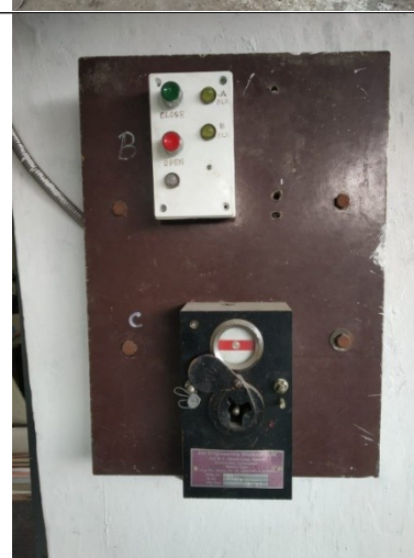
LC gate no.10T at BBDB of Sealdah division.
