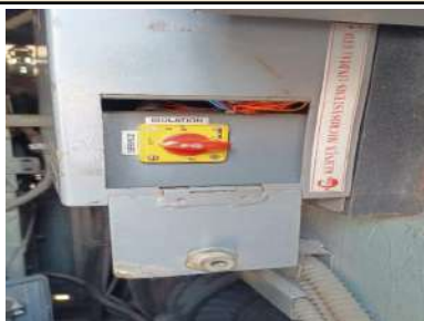
Fig. 18(12) Kernex: Kavach Isolation switch
