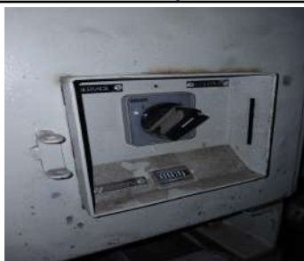
Fig. 18(11) HBL: Kavach Isolation switch at BIU unit
