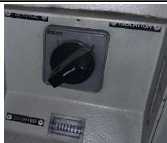
Fig. 18(13) HBL: Kavach Isolation switch at BIU unit
