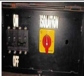
Fig. 18(14) Medha: Kavach Isolation switch at onboard kavach
