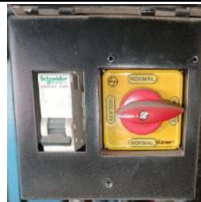
Fig. 18(10) Medha: Kavach Isolation at onboard kavach
