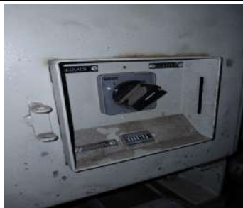
Fig. 18(11) HBL: Kavach Isolation switch at BIU unit
