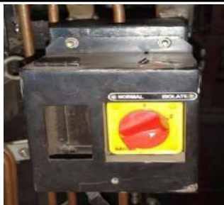
Fig. 18(9) Kernex: Kavach Isolation switch at Pn. panel
