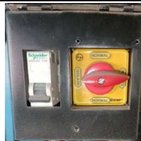
Fig. 18(10) Medha: Kavach Isolation at onboard kavach
