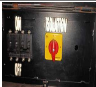
Fig. 18(14) Medha: Kavach Isolation switch at onboard kavach
