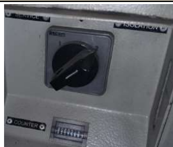
Fig. 18(13) HBL: Kavach Isolation switch at BIU unit
